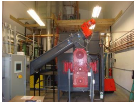
Boiler 3 MMBtuh Hot Water 500 lb/h 25% Char
